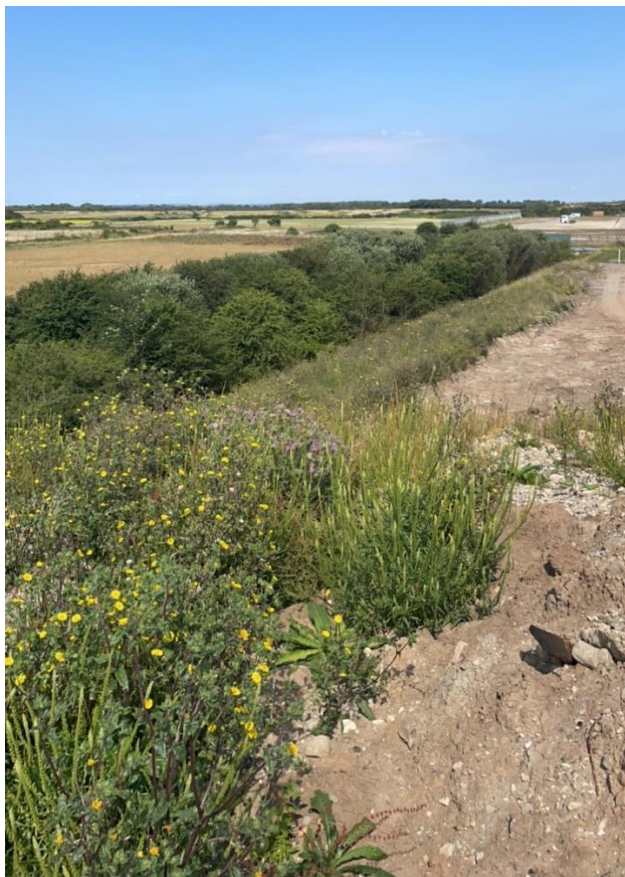
Photograph 7. Wet ditch with steep earth banks and overgrown vegetation.
