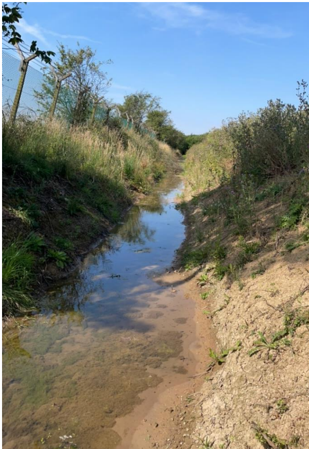
Photograph 6. Wet ditch with steep earth banks and overgrown vegetation.
